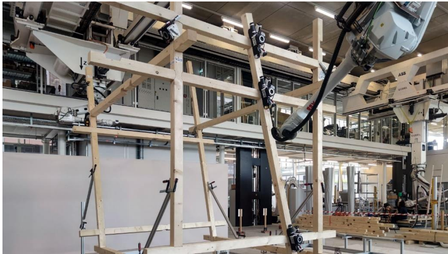
Fig. 9. Image of a beam being assembled by screwdrivers. Note that some clamps remained on the structure from the previous assembly.
