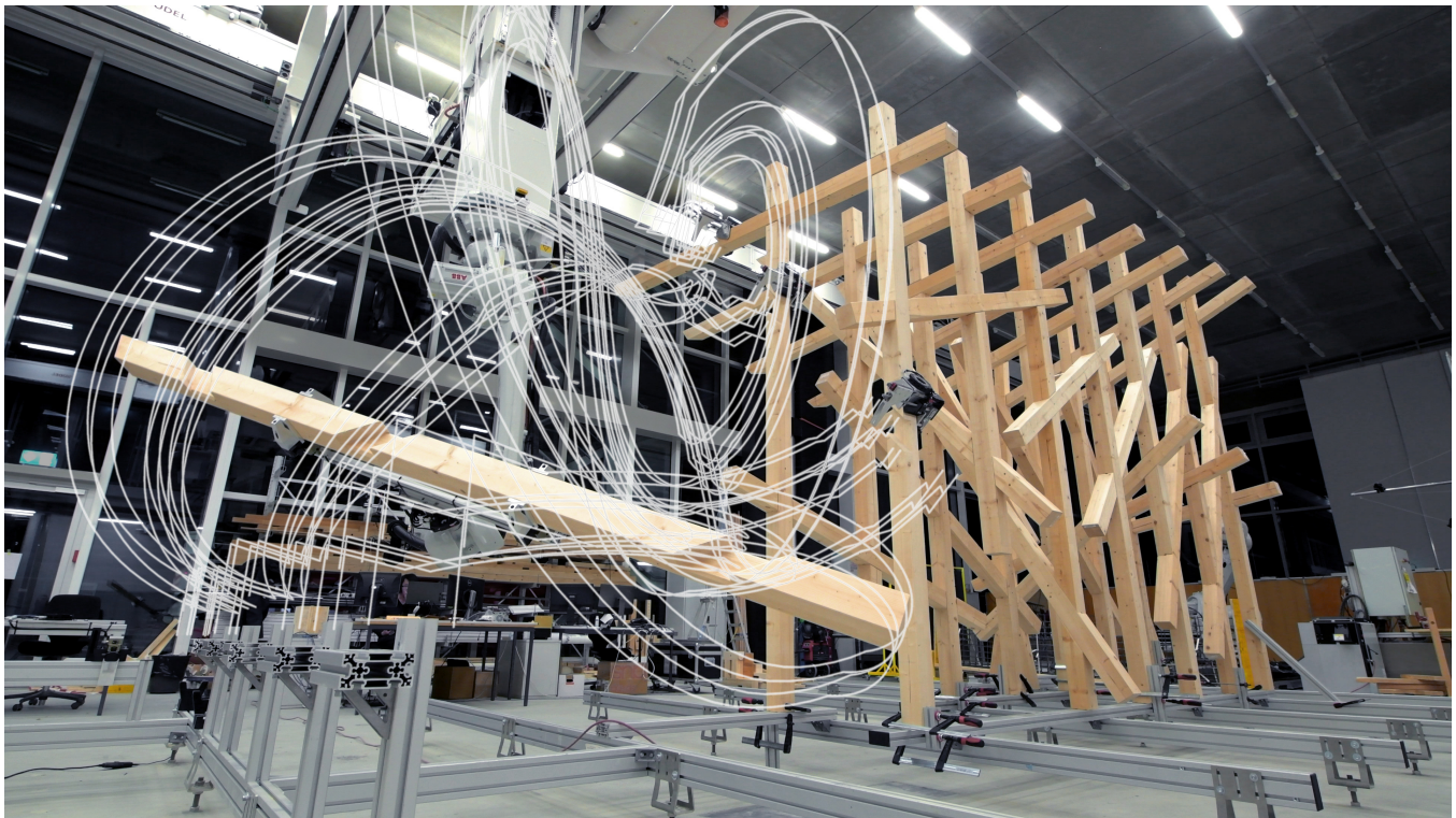
Figure 1: Image showing the final timber element being assembled in our case study. Three distributed clamps can be seen in the background already attached to the structure by the robotic arm. The assembly process is modeled with our flowchart and solved using our solver. Two linear and one free motion trajectory are used to bring the element from pickup to the clamps, shown here as overlaid white curves.
