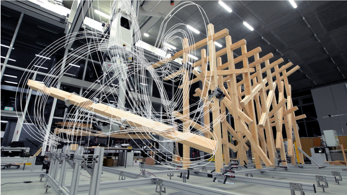
Figure 5-1: Image showing the final timber element being assembled in our case study. Three distributed clamps can be seen in the background already attached to the structure by the robotic arm. The assembly process is modeled with our flowchart and solved using our solver. Two linear and one free motion trajectory are used to bring the element from pickup to the clamps, shown here as overlaid white curves.
